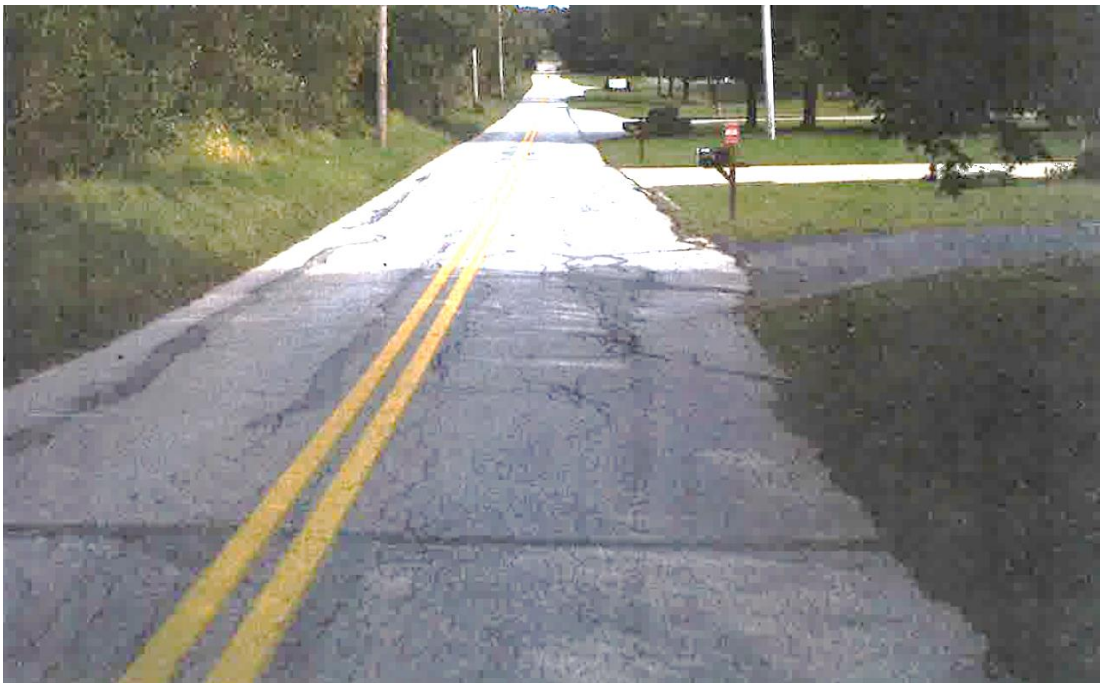
Figure 11: Example of local hot mix pavement in very poor condition with OPC 7.6
