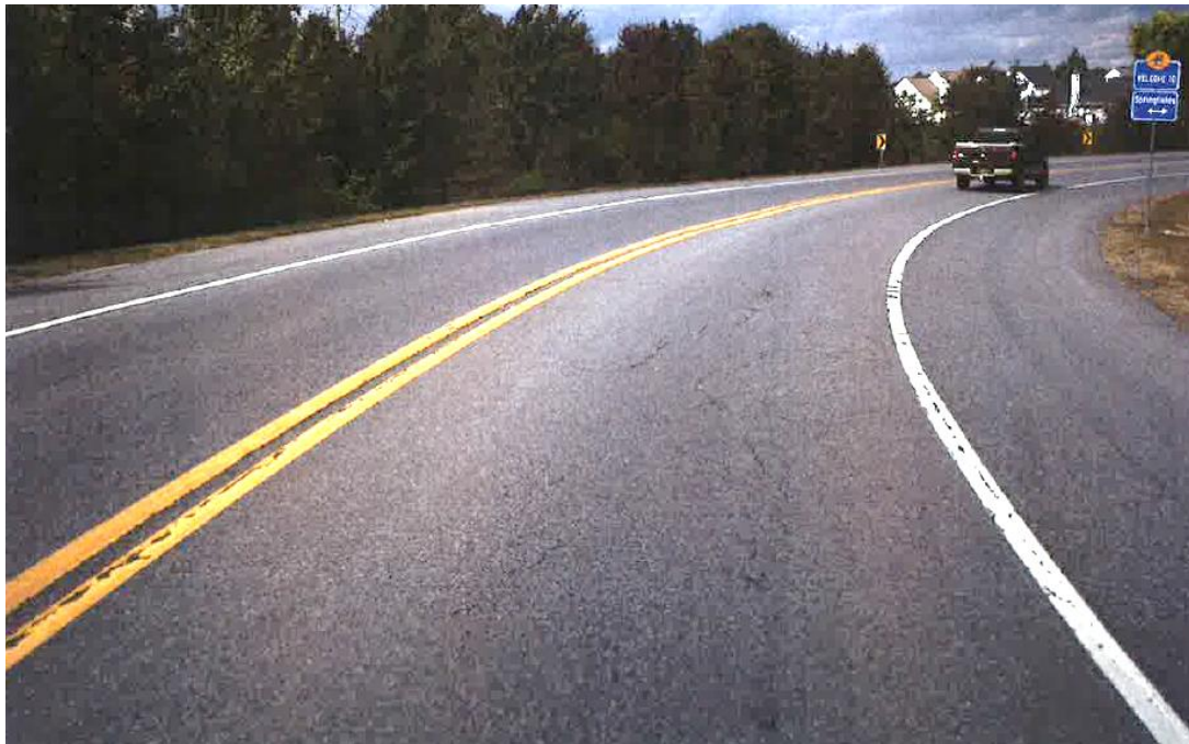
Figure 9: Example of major collector hot mix pavement in fair condition with OPC 58.2
