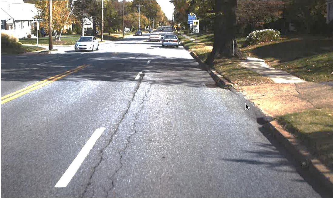
Figure 10: Example of major collector composite pavement in poor condition with OPC 48.6
